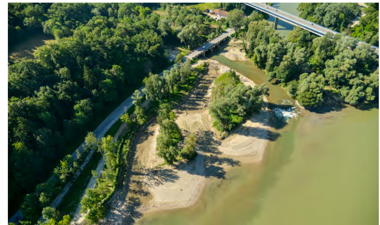
Fig. 5: Mouth of the Pielach – redesign of the river mouth and construction of a nature conservation area. © Markus Haslinger
